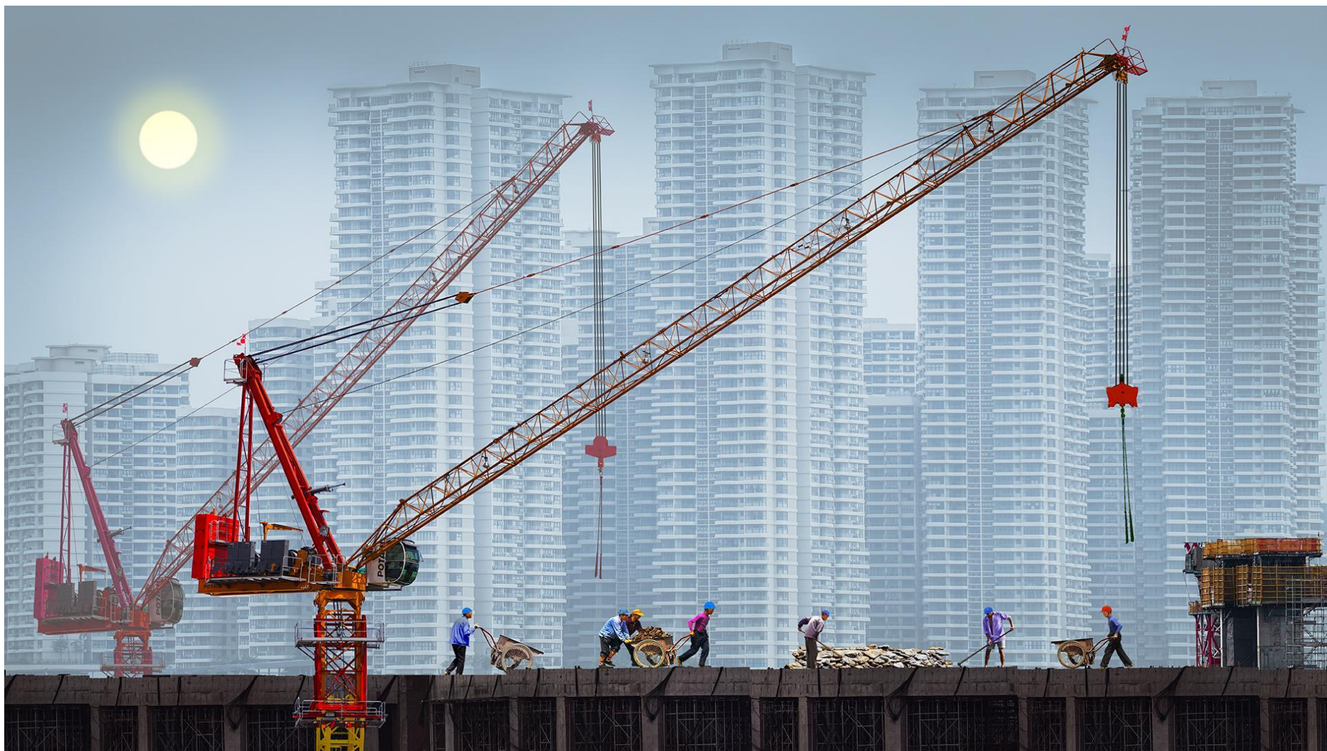
Honourable Mention | Judging 2 | Pixelite International Circuit 2023 | COLOR OPEN (PIDC) (DIGITAL) | The Song Of Construction Sites 4 | Kim Yiang CHNG | Singapore
